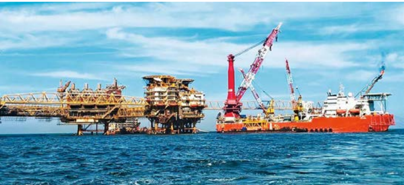
Additional development of Vasai East Project for ONGC. The scope included EPCIC of 2 wellhead platforms, 35 km pipelines and modification.
