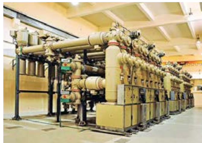
One of the many 400 kV Gas-insulated Substations installed by L&T.
