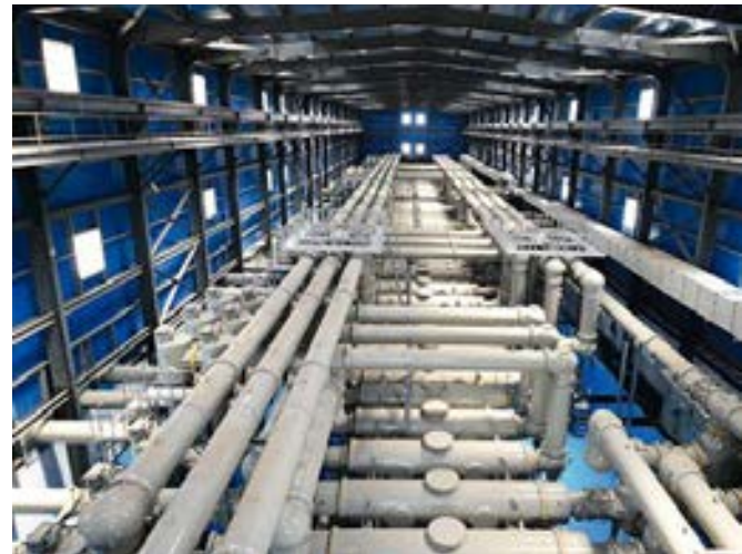
765 kV Gas-insulated Substation, Varanasi.
