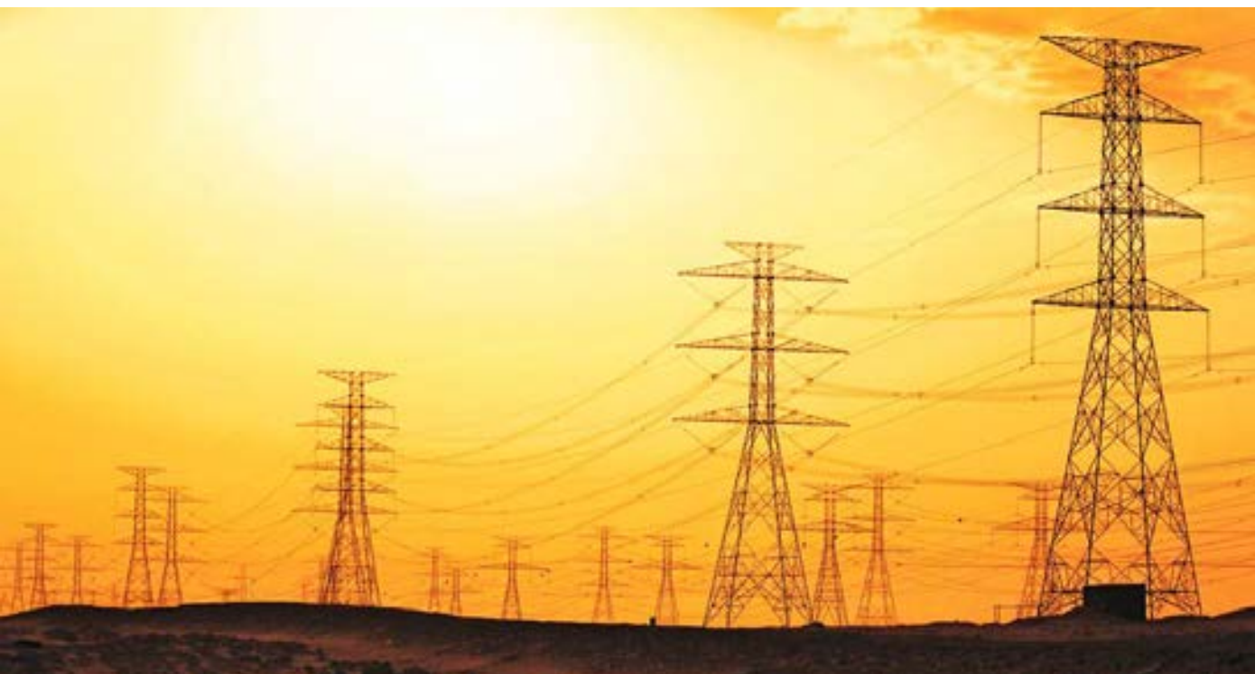
230 kV double circuit transmission line at Abu Ali, Saudi Arabia.
