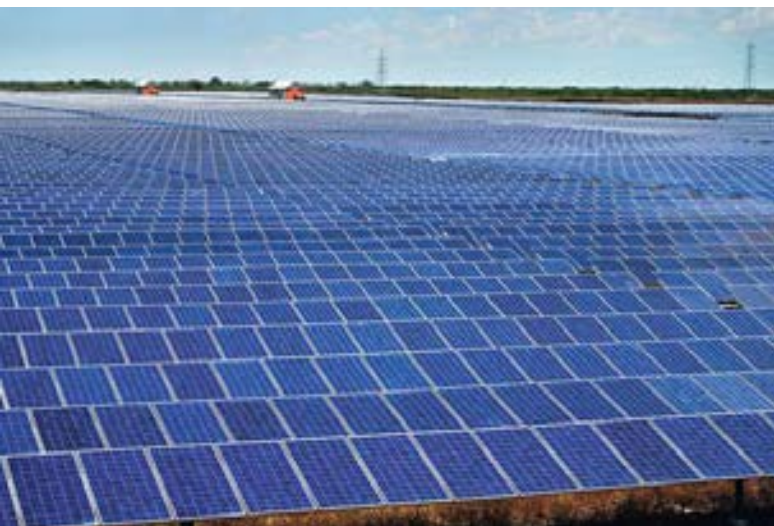
60 MWp Solar Tracker Plant, Tamil Nadu
