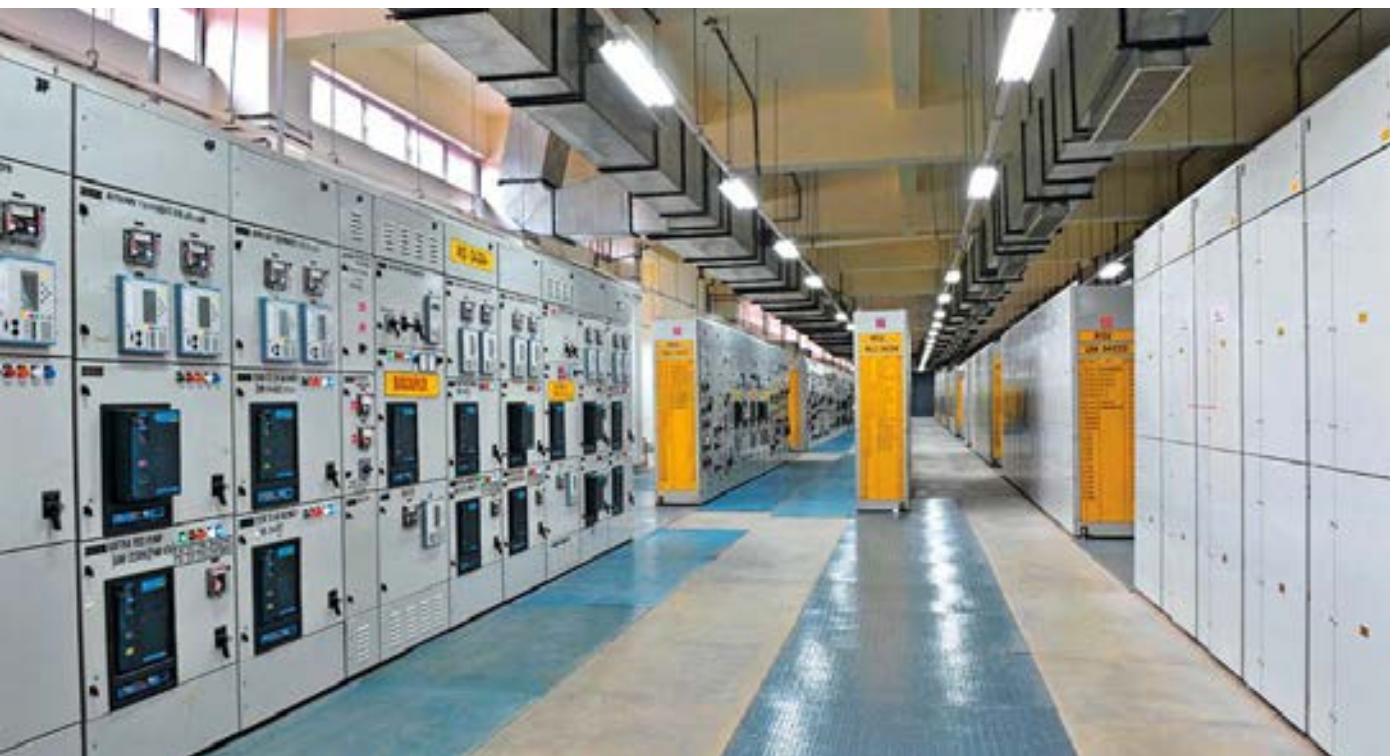
Switchboard installation at a power plant. L&T provides power distribution and control solutions across the value chain, from generation to end user.
