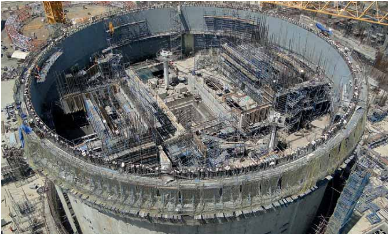
Kakrapar Atomic Power Project, Gujarat, under construction. L&T has contributed to India's nuclear power programme both through comprehensive construction of critical structures and supply of vital equipment.
