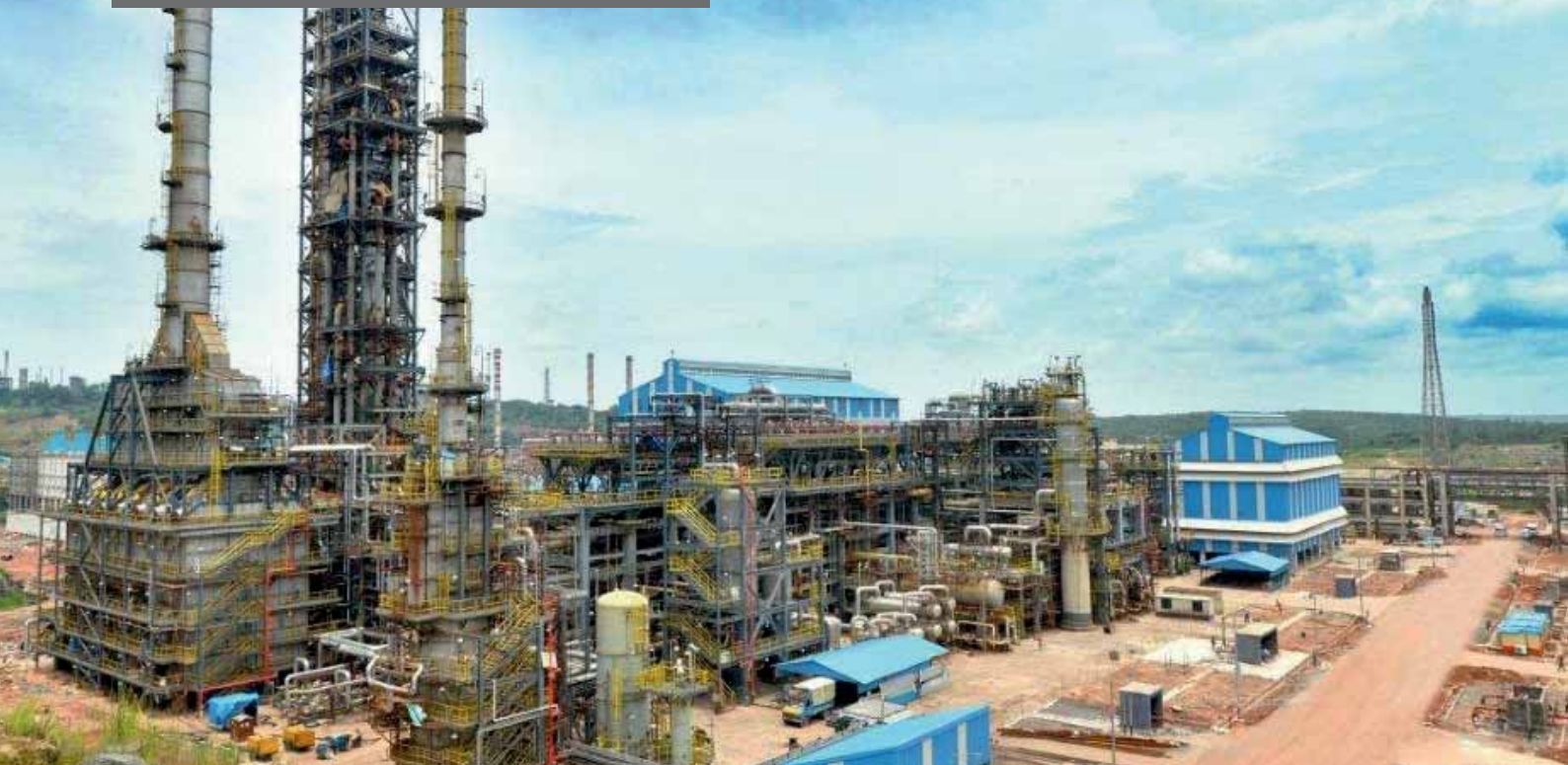
Aromatic Complex built on LSTK basis for ONGC Mangalore Petrochemicals Limited.
