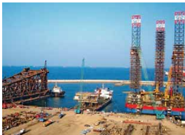
A jack-up rig along with a wellhead platform and a jacket at L&T's Modular Fabrication Yard in Sohar, Oman.
