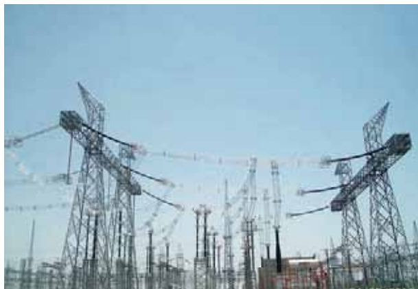
India's first 1200 kV substation at Bina in Madhya Pradesh built by L&T.
