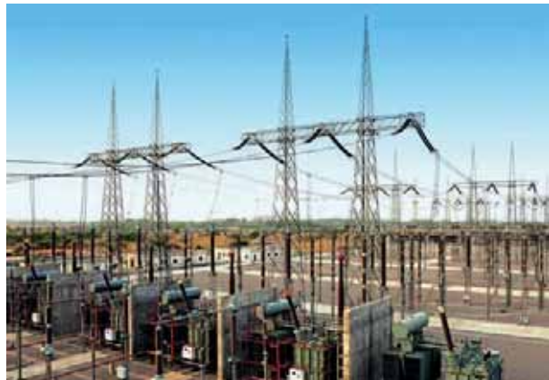
Substation incorporating 765 kV Air-Insulated Switchgear at Unnao in Uttar Pradesh. L&T offers complete solutions in high-voltage substations and power transmission lines.
